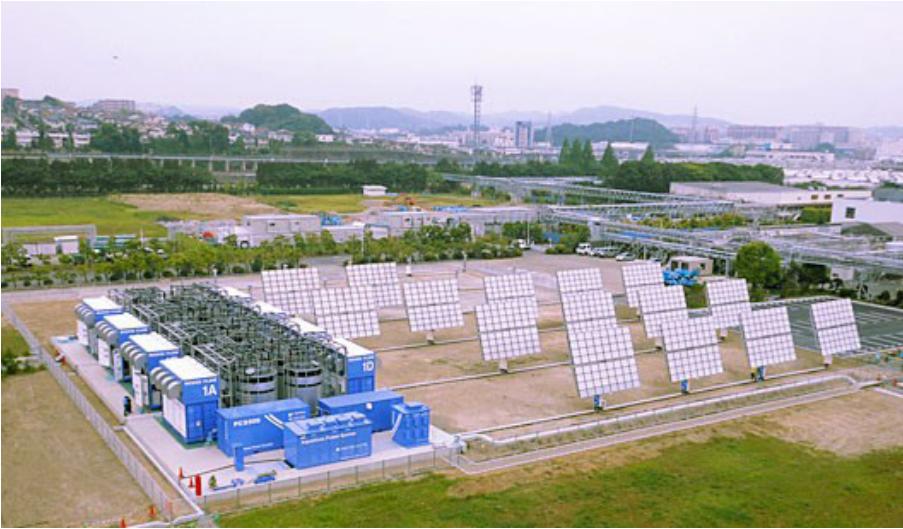
Fig. 5. — PV and batteries project.
