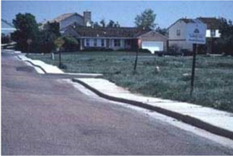
Fig. 5. — Effect of differential heave on roads and infrastructure.
