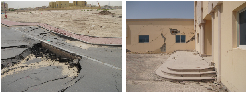
Fig. 16. — Effect of subsidence due to dissolution of salt on infrastructure (left) and buildings (right) (UAE).
